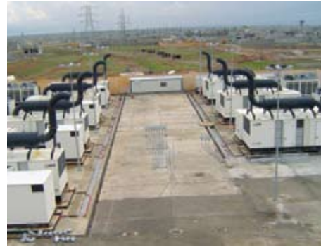
Seven enclosed gen sets providing continuous power to homes and businesses in Northern Iraq
