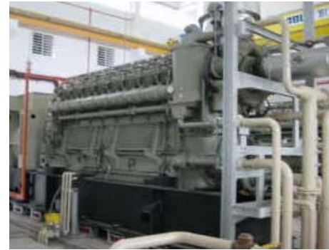
Unenclosed gen set for a water treatment plant in Indonesia
